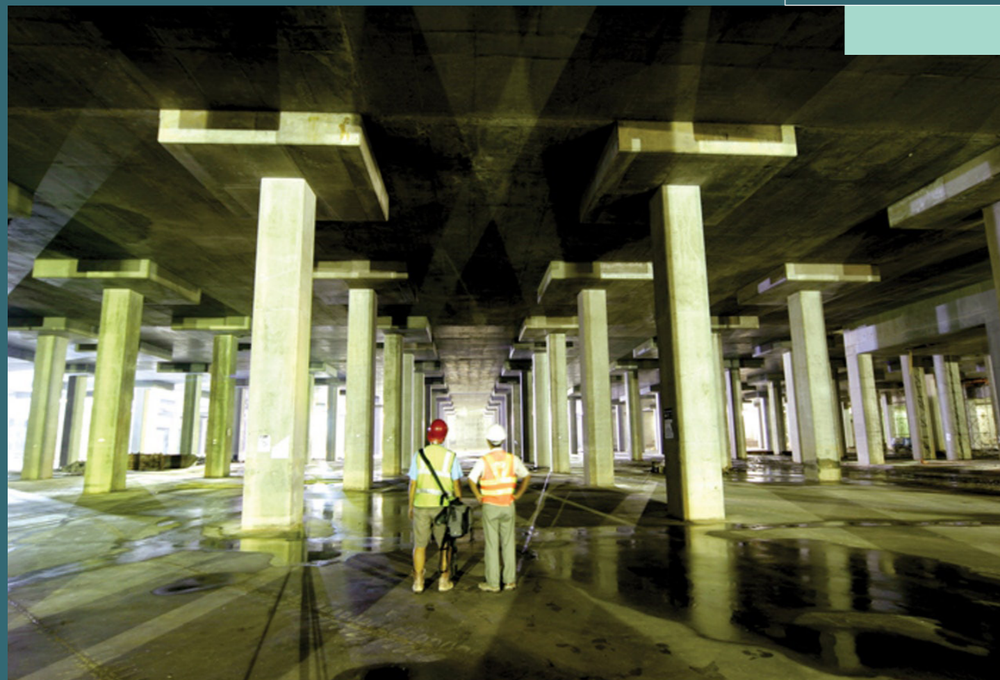
Tai Hang Tung Stormwater Storage Tank. Source: Drainage Services Department.
